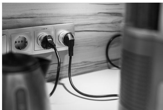
(b) appliances with attached power meters
